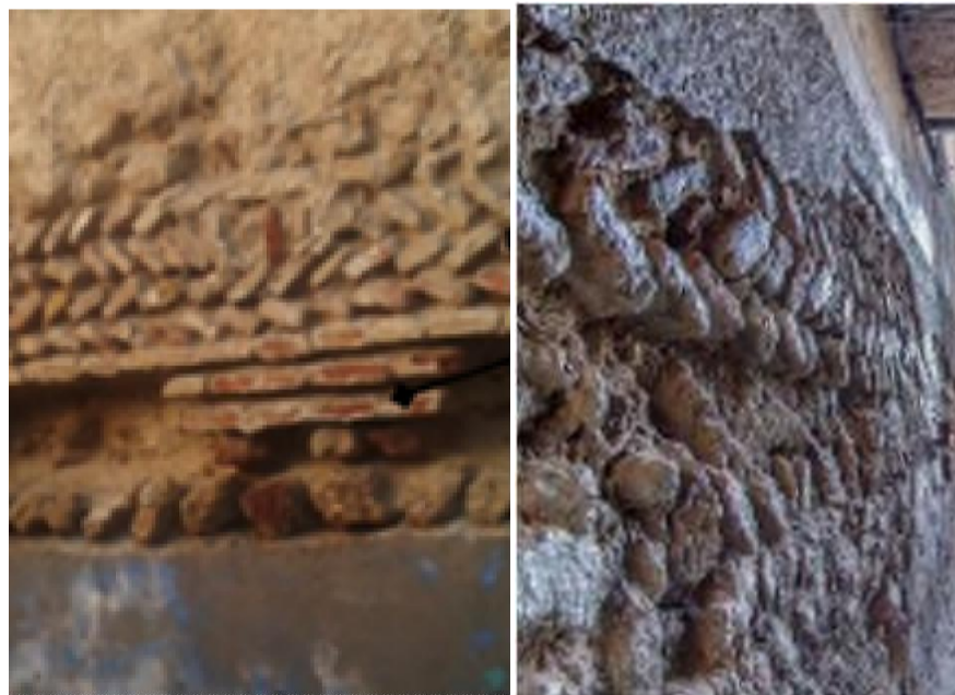
Fig. 3. Mixed walls with double layer of terracotta brick and rubble-medina of Tlemcen.
